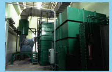
Odor & Dust Control System
