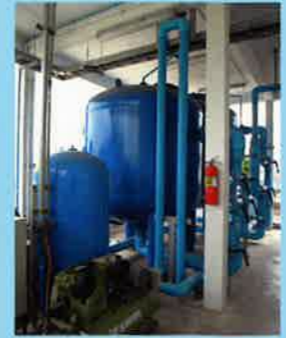
Refuse Water Filter
