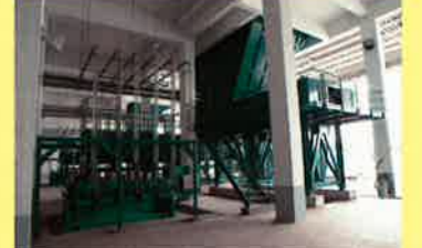
Hydraulic Power Unit
