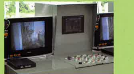
Central Control Panels
