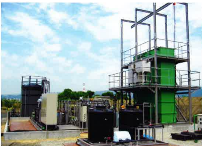
Demonstration plant for Low Power Consumption Desalination System
