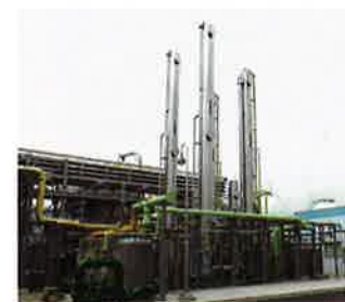
Biogas upgrading system
