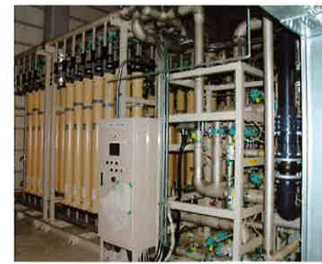
Membrane Separation System
