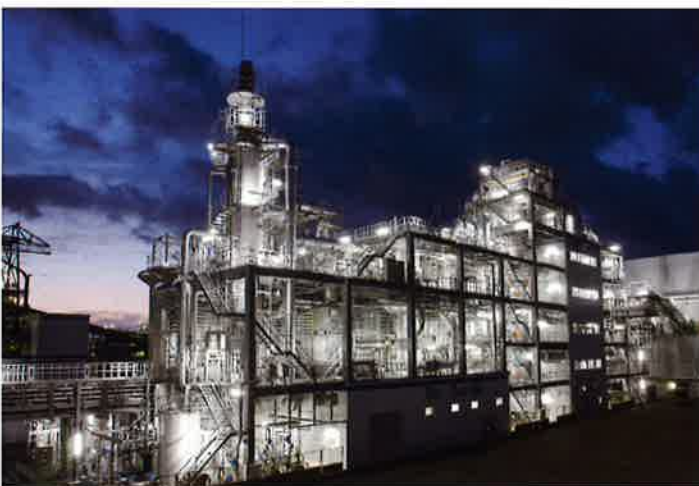
Advanced Two-stage Incinerator
