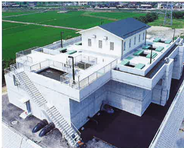
Upper counterflow type biological contact filter, U-BCF
