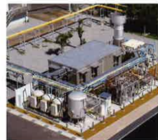
Biogas purifying technology for the injection into the city gas grid
