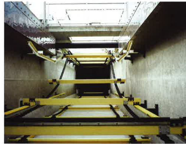
Non-metallic sludge-gathering system
