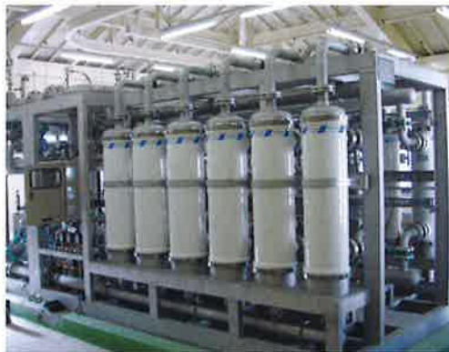
Ultra membrane filtration system
