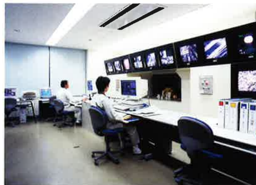
Central control room
