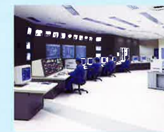
H Central control room
