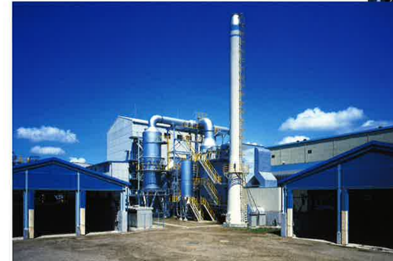
Funabashi Clean Center, Kanematsu, Chiba 75 tons/day × 2 furnace units for construction waste including waste plastics and wood, etc., completed in 1994.
