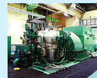
G Steam turbine generator room
