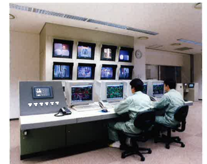
Central control room
