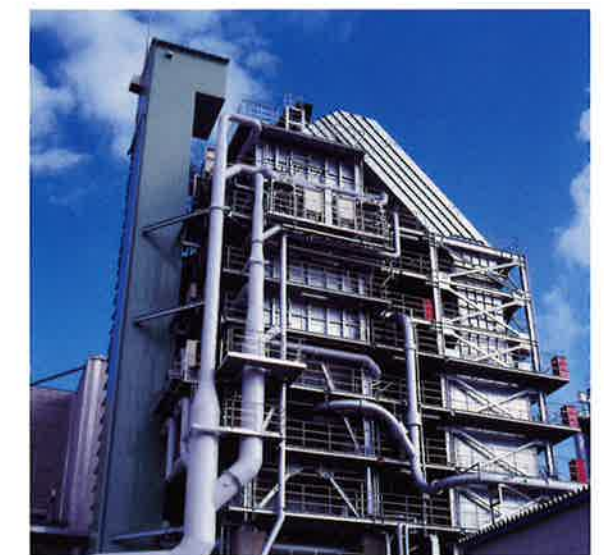
Motomachi Environment Center 160 tons/day × 1 furnace, for general industrial waste, plastics, vinyl, rubber, sludge, waste/chemical oil, paper, etc., completed in 1997.
