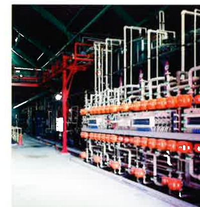
Water treatment system
