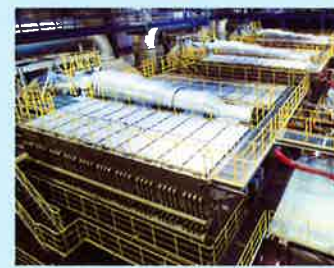
E Flue gas treatment system
