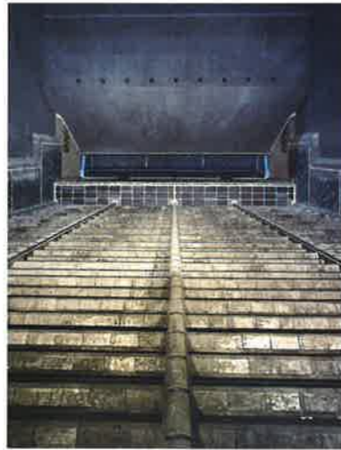
Stoker type refuse incinerator*1
