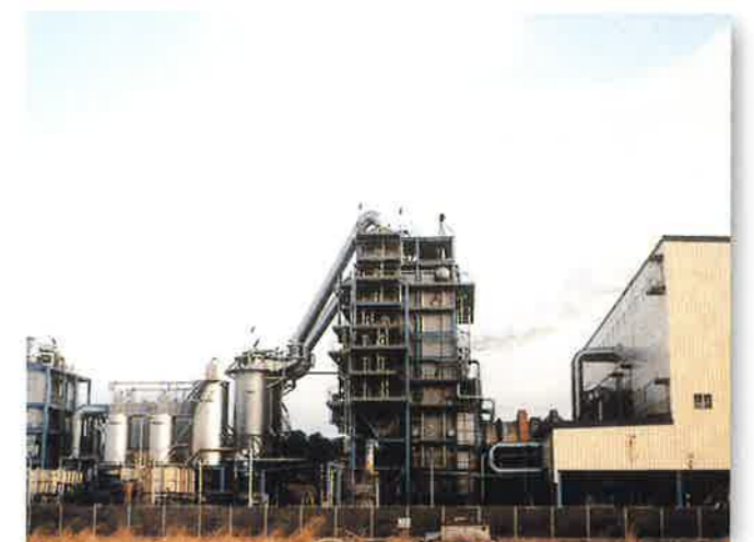
■ Kashima Joint Resource Recovery Center <Completed March 2001> Rotary kiln type incinerator (Treatment volume: 100t/day x 2 furnaces, Power generated: 3,000kW)
