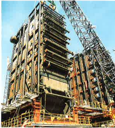
High efficiency refuse burning power generation system *4
