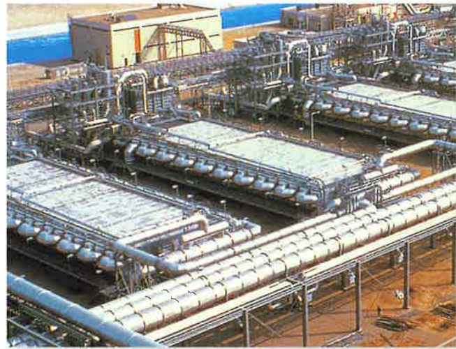
■ Saudi Arabia Desalination Foundation Al Khobar <Completed March 2001> (Treatment capacity: 35,000m 3 /day x 8 systems)
