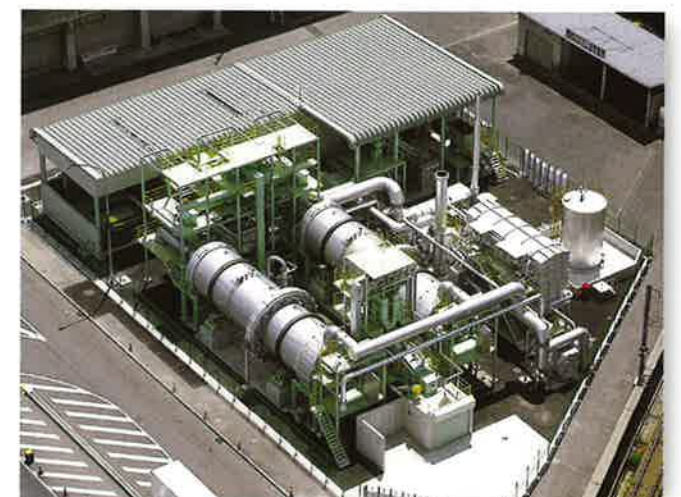
■ Osaka Prefectural Central Wholesale Market, High speed garbage-to-resource conversion system <Completed August 2001> (Treatment volume: 50t/day)
