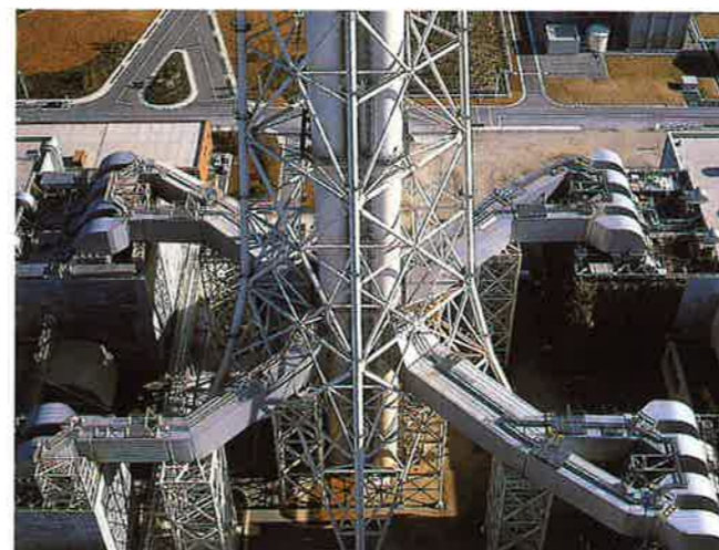
■ Tokyo Electric Power Company, Futsu Power Generation Plant, Selective catalytic reduction (De-NOx Facility) <Completed February 2000> (Treatment capacity: 1,250,000Nm 3 /h x 14 systems)
